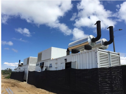
Colombia power Diesel plant project
