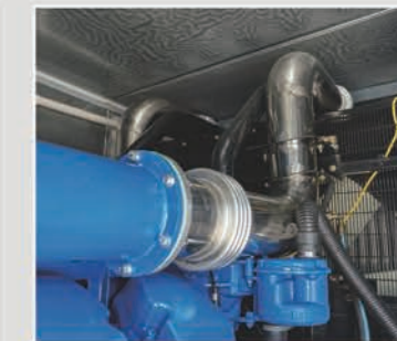
Interior of the genset
